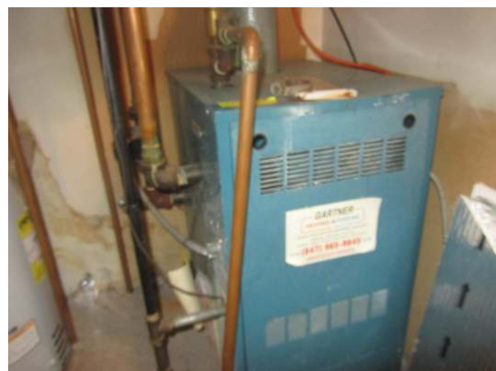
Boiler in closet is past typical life of 20-25 years 1989 MFD .
