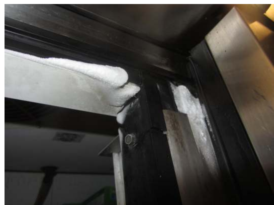
Frost/seal break at wall freezer doors
