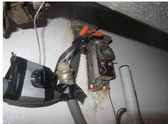
Exposed electrical within walk-in at compressor
