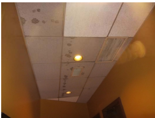
Past ceiling stains in hall, source in unknown
