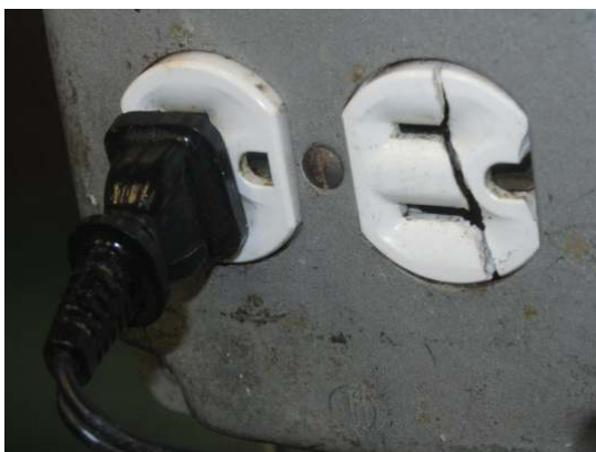
Damaged outlet at walk-in exterior Wall/prep counter
