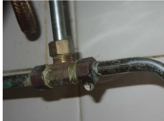
Minor water leak at hand sink in kitchen
