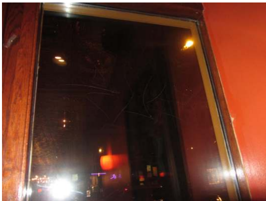
Storefront window scratched/graffiti
