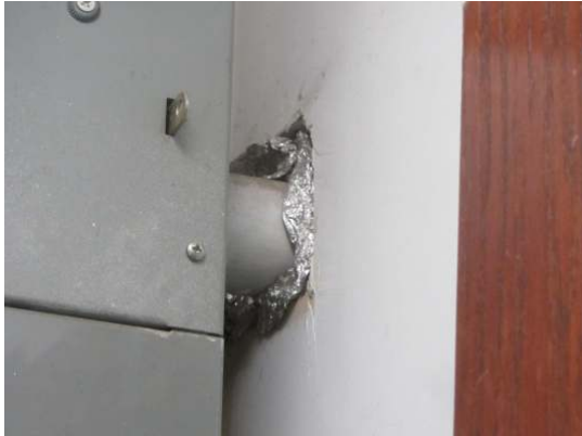
Suggest properly sealing air gaps at Main power to avoid rodent risk
