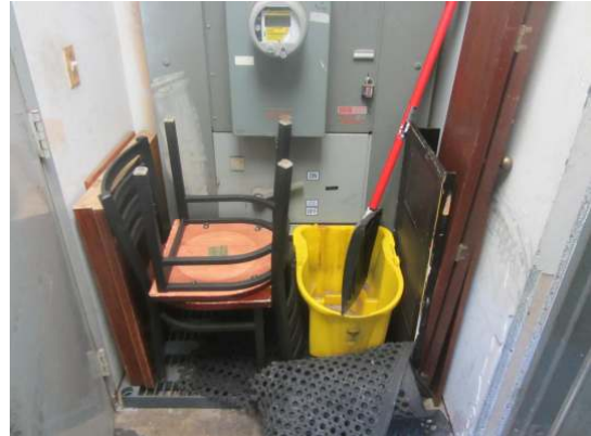
Suggest maintaining proper clearance to power main.
