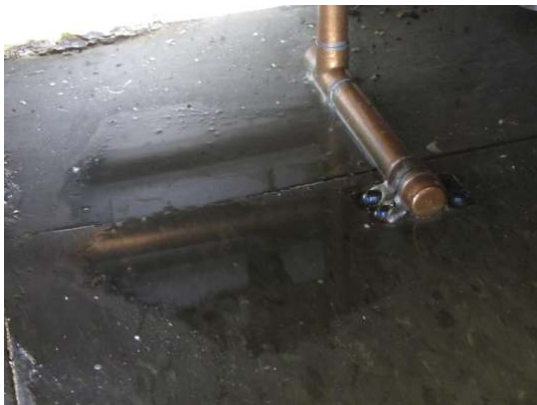
Standing water under line and dishwasher
