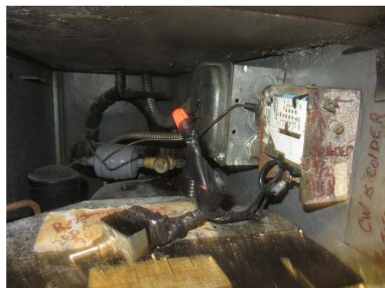
Exposed switch wiring at line cooling
