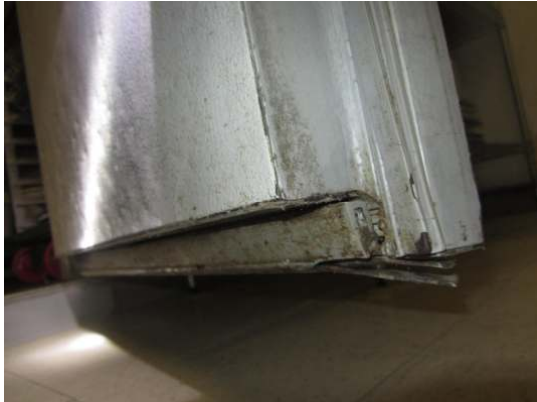
Main walk-in door seal slightly torn
