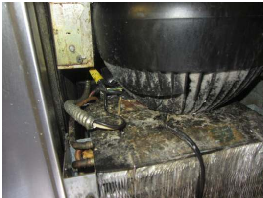
Exposed high voltage wiring at line Cooling compressor
