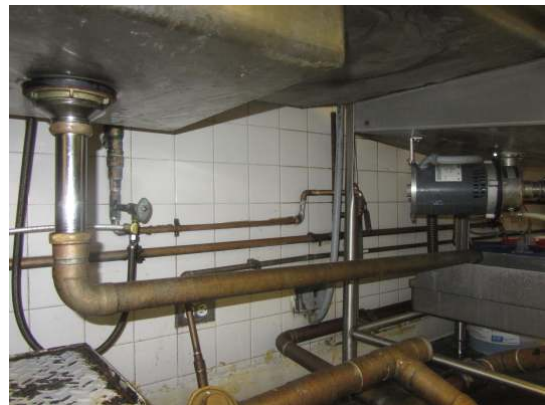
Loose drain pipe at dishwasher
